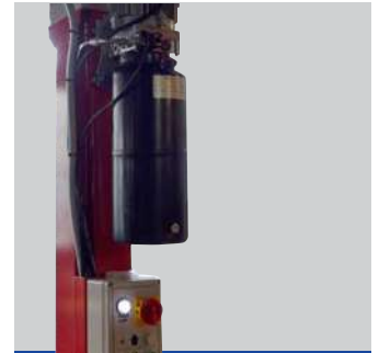
Control Unit / Pump
